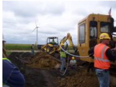
Underground Collector Line
